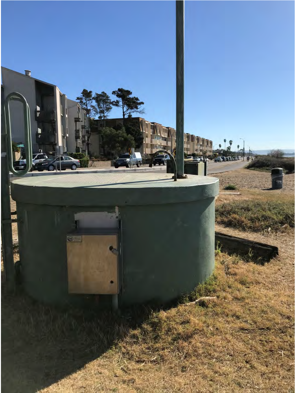
Figure 3B –Lagoon Intake Pump
