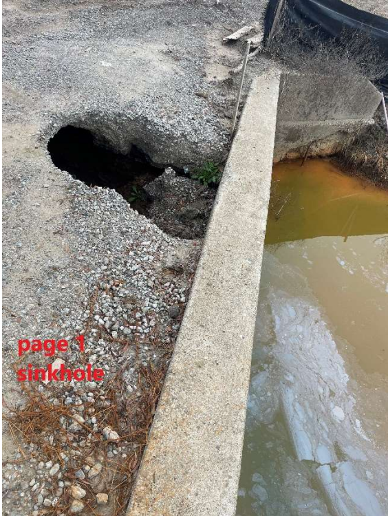
Figure 22 – Sinkhole in 36” PVC Culvert Just Upstream of the Golf Course SDPS Retention Pond on the East Slough
