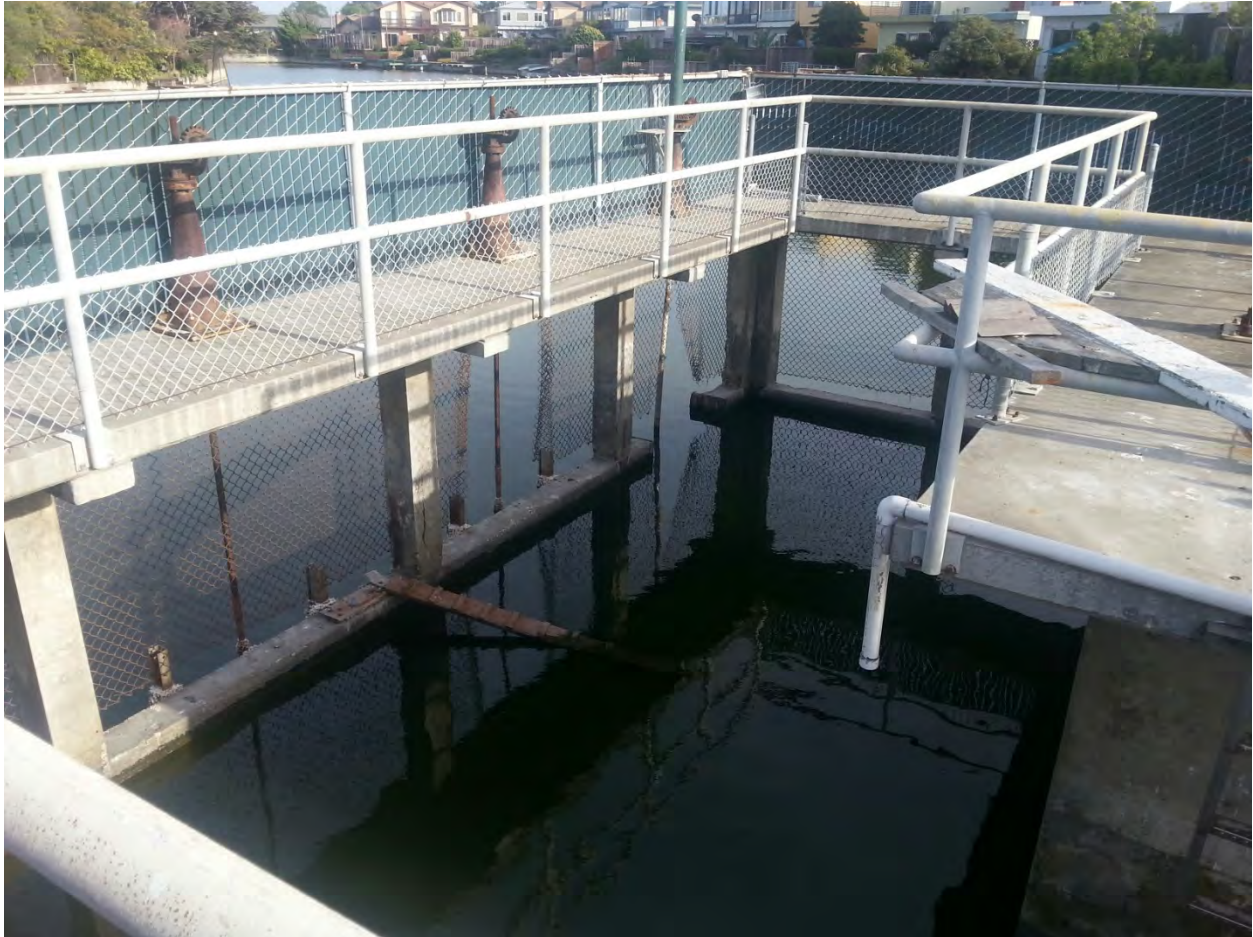
Figure 5B –Lagoon Outlet Condition
