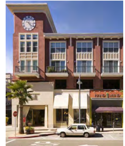
Corner volume encroaches into setback area.
