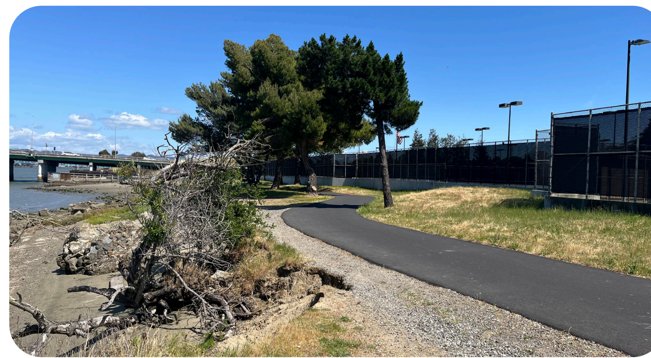
Tree fall at erosion in front of Harbor Bay Club
