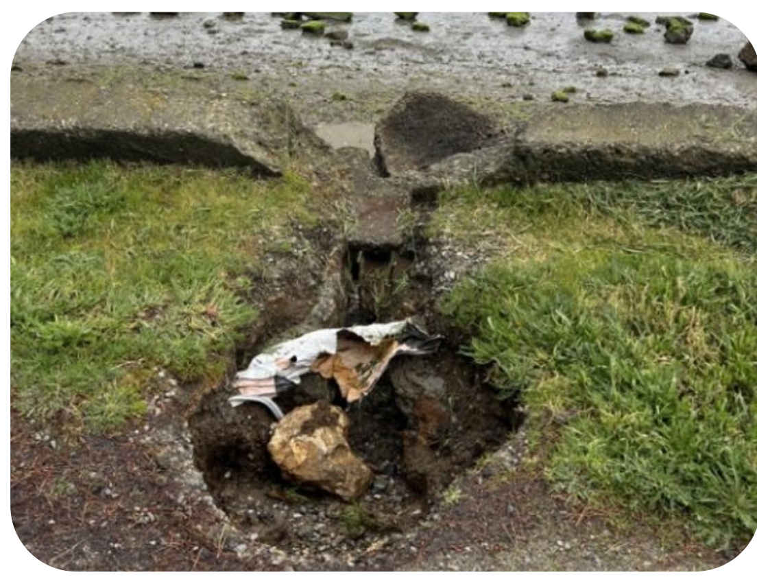
Erosion at stormwater runoff outlet pipe
