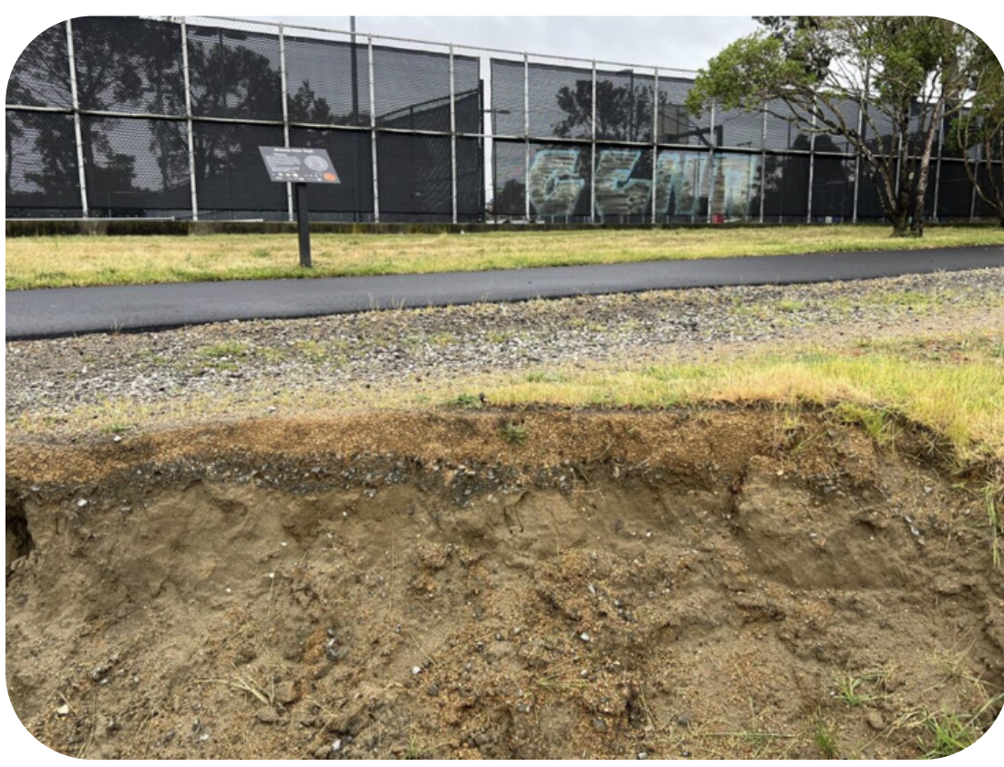
Erosion adjacent to Bay Trail next to Harbor Bay Club
