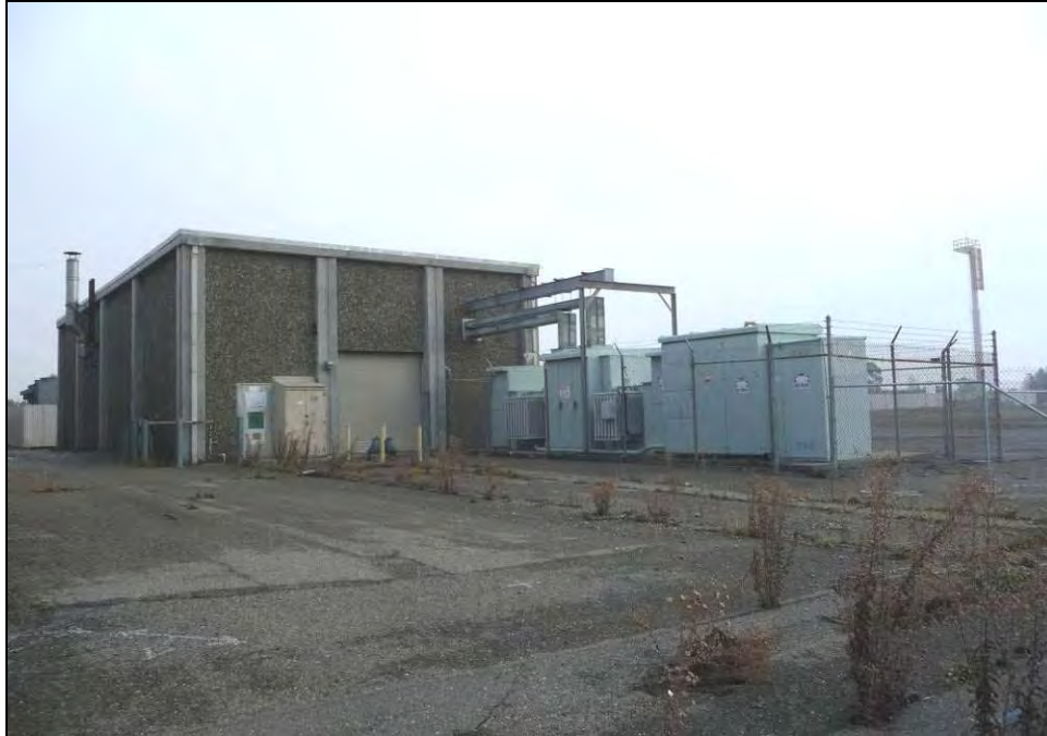
Photograph 4: Building 529, substation equipment, camera facing southeast, December 16, 2009.
