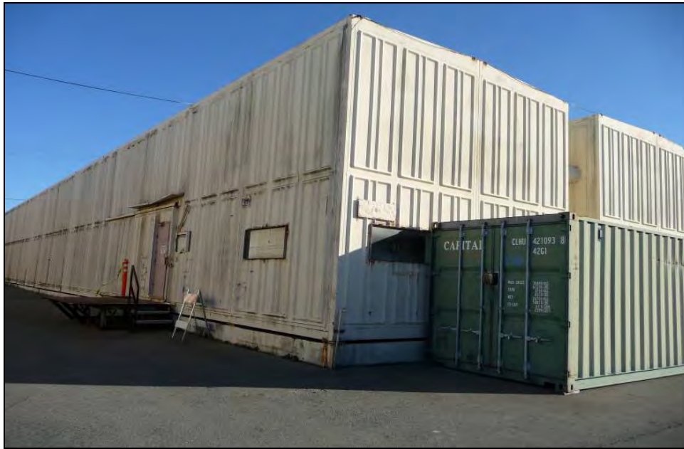
Photograph 3: Buildings 338A-H, stairs leading to personnel door, office windows on the north and west side, camera facing southeast, December 22, 2009.
