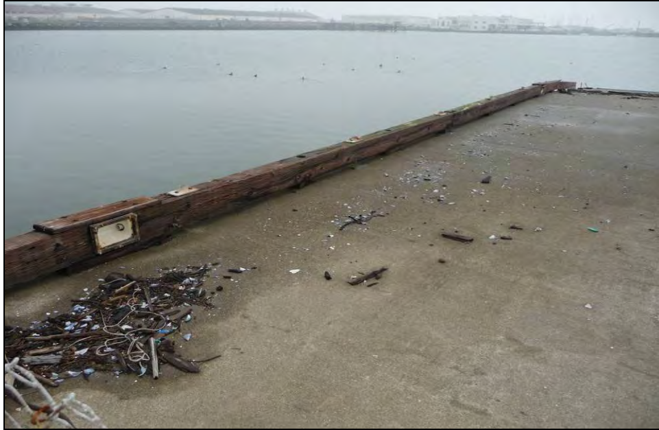
Photograph 14: Wooden bumpers with metal posts of Dock 4 running along eastern side of Ramp 4, camera facing southeast, December 16, 2009.
