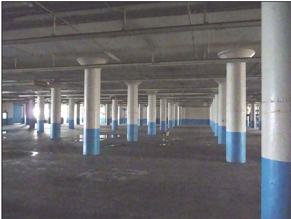
Photograph 4: Interior of Building 8, showing open space with support piers, camera facing east, December 16, 2009.
