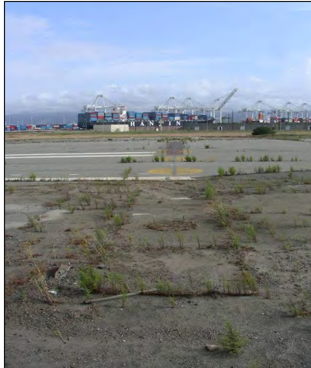
Photograph 8: Remnant of emergency arresting gear on Runway 13-31, camera facing north, October 14, 2009.
