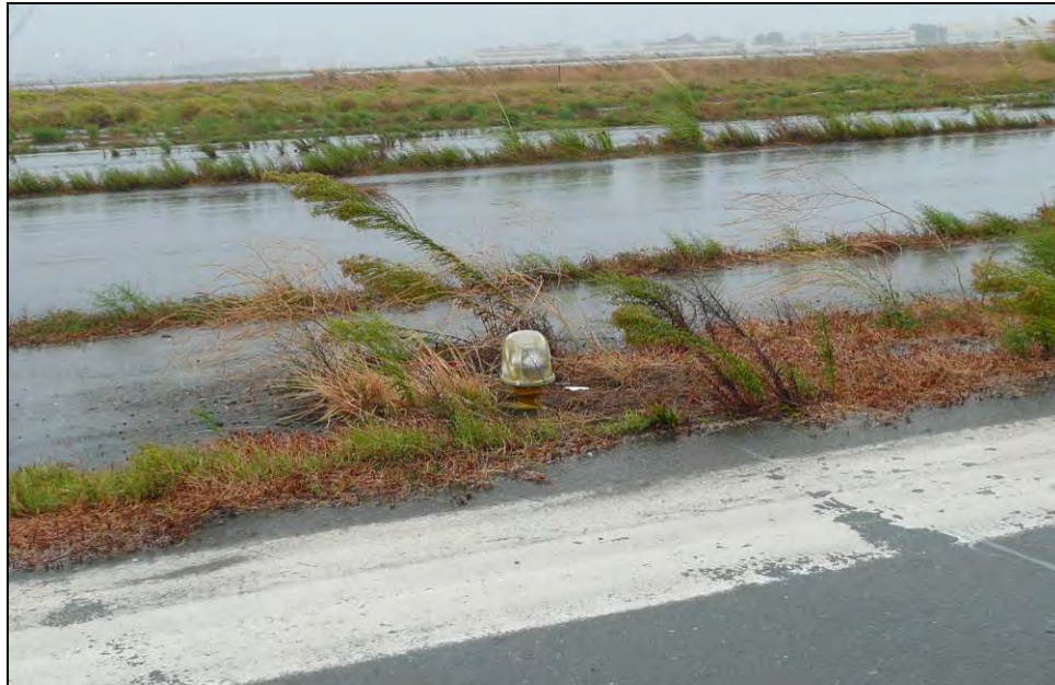
Photograph 6: Rotating runway light along edge of Runway 13-31, camera facing southeast, October 13, 2009.
