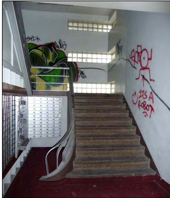
Photograph 7: Interior of Building 17, showing terrazzo flooring on steps, curved staircase and handrails, and glass block window elements, camera facing north, December 11, 2009.
