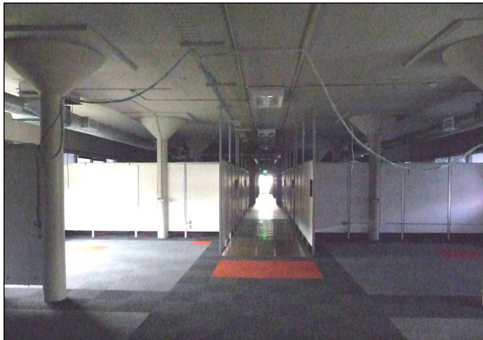
Photograph 14: Showing cubicle partition in dormitory and distinctive “mushroom” style concrete supports, Building 2, camera facing north, December 11, 2009.
