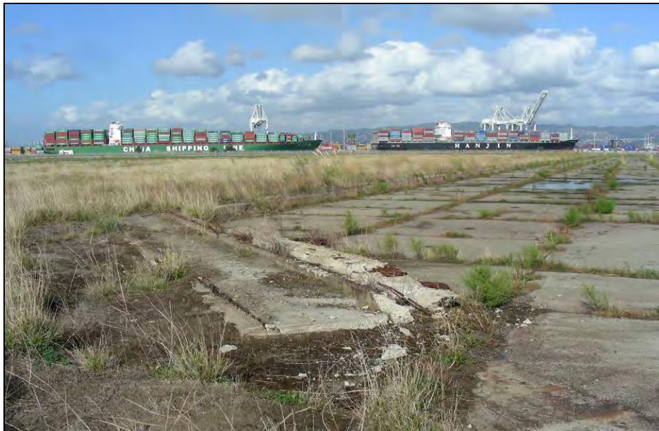
Photograph 19: Detail view of remnant curb of concrete apron near Taxiway F, camera facing northwest, October 14, 2009.
