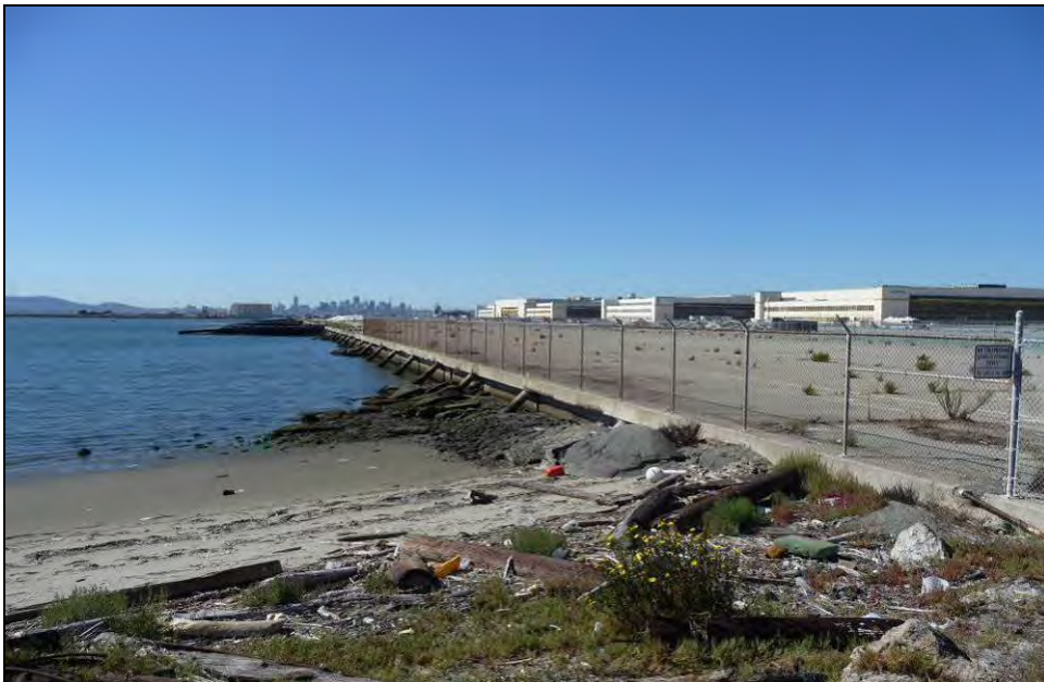
Photograph 5: Seaplane Lagoon, northeast corner, Ramp 4, northern bulkhead (Building 200648) and concrete apron north of Seaplane Lagoon visible, Seaplane Hangars at right, camera facing west, October 1, 2009.
