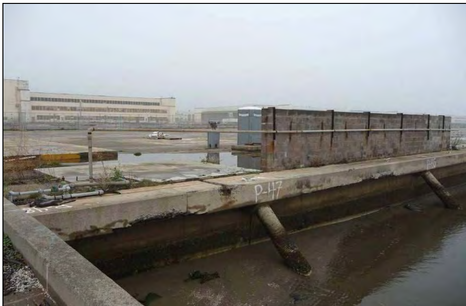
Photograph 15: Area adjacent to Ramp 1, showing northern bulkhead, concrete apron, and concrete support pylons, camera facing northeast, December 16, 2009.
