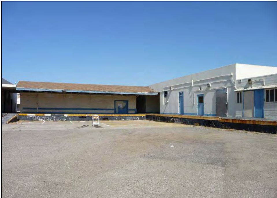
Photograph 6: Loading dock area on west side, connecting addition on the left, camera facing northeast, October 6, 2009.
