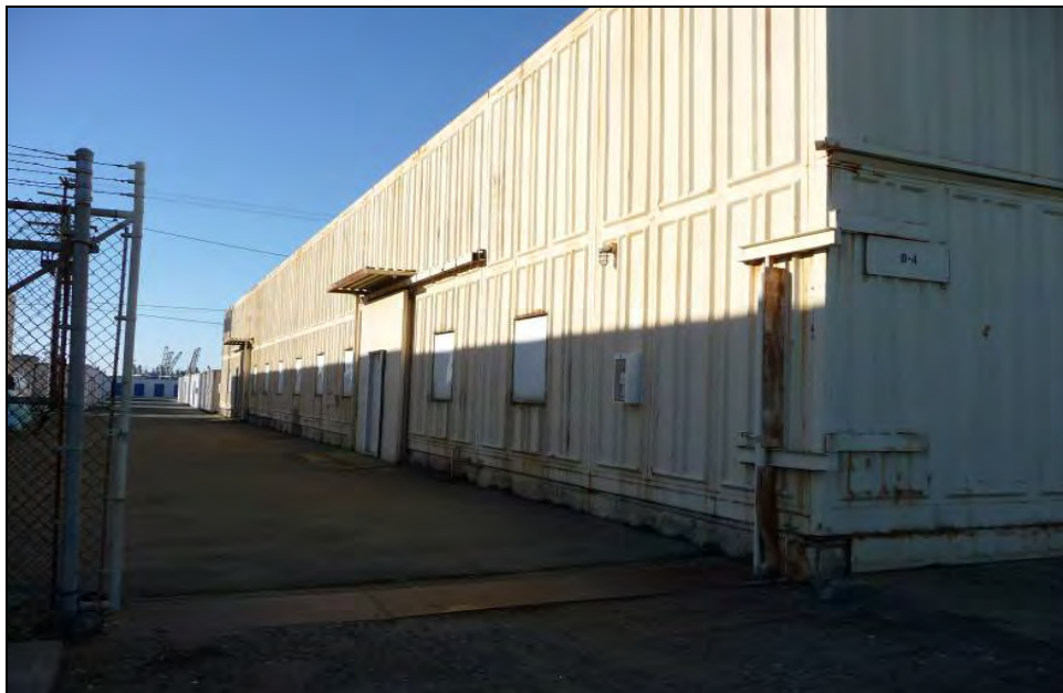
Photograph 4: Buildings 338A-H, personnel door and office windows boarded, camera facing northwest, December 22, 2009.
