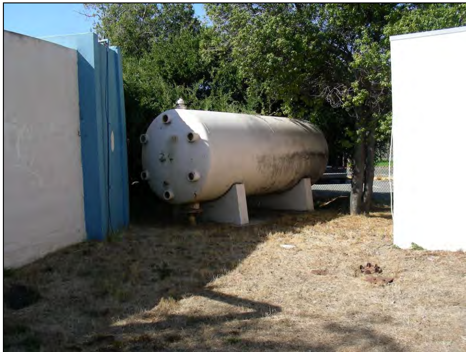
Photograph 3: Metal tank on northeast side of Building 95, camera facing northwest, September 29, 2009.
