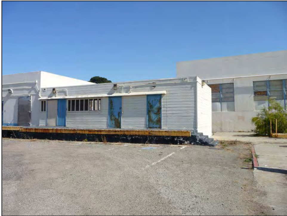
Photograph 7: Wooden addition to south of food storage wing, camera facing east, October 6, 2009.
