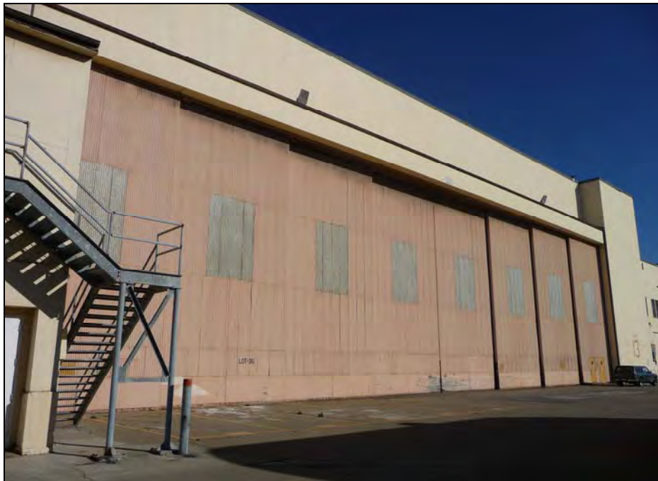
Photograph 4: Door 13 on the west side showing flat parapet of the side doors of the Interim Overhaul area, camera facing southeast, September 29, 2009.
