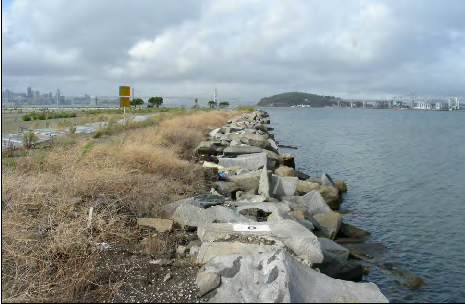
Photograph 2: Portion of seawall along northern edge of Airfield, camera facing northwest, October 14, 2009
