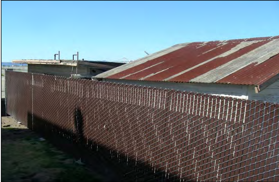
Photograph 14: Unnumbered wooden structure to the west of Building 377A, camera facing northwest, September 30, 2009.
