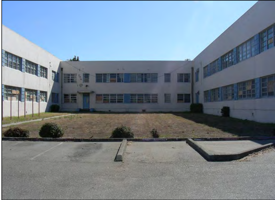
Photograph 5: Non courtyard elevation of connecting element between Wings 18 and 19, Building 4, camera facing south, October 7, 2009.
