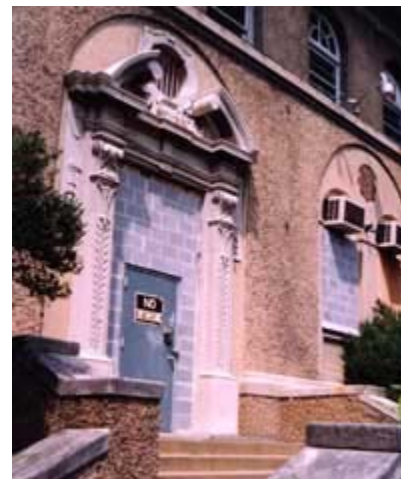
The first floor openings of this historic building have been filled with cinder blocks and the doors, window sash, and frames removed for safe keeping. The security metal door features heavy duty locks. Photo: NPS files.
