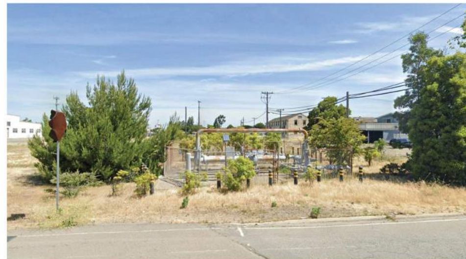
2. PG&E GAS FACILITY
